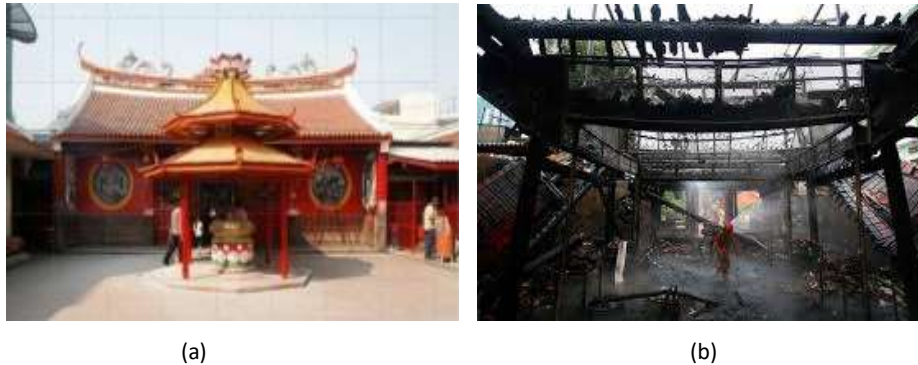
Figure 1 Condition of Dharma Bhakti Monastery: (a) before and (b) after burning.
