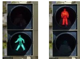
Figure 1. Pedestrian Traffic Light
