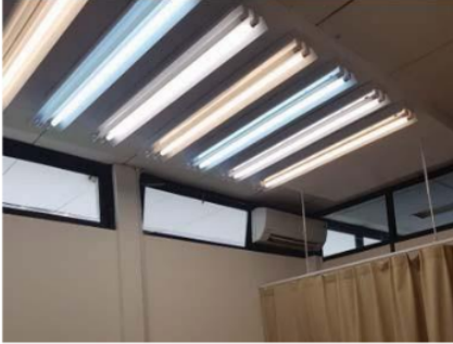
Fig. 1. The lighting system arrangement with 3 types of illumination.
