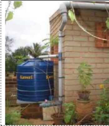
Figure 1. Rainwater collection tank on the ground surface (source: www.hyderabadwater.gov.in )
